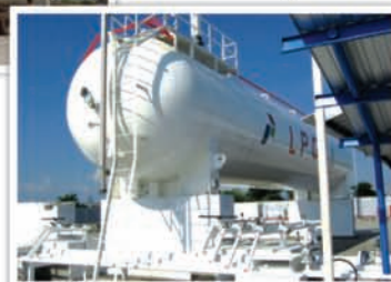
Tanki LPG 30 Ton Project SPPBE Pertamina Jember
